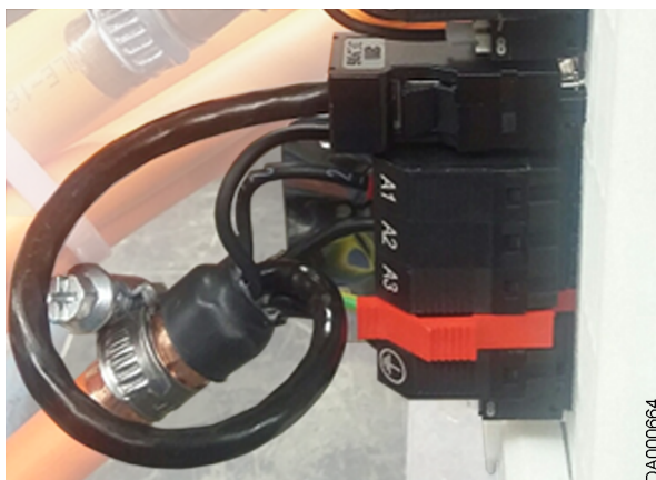
Fig. 52: Encoder cable forming a loop to be led to connection point XG20
