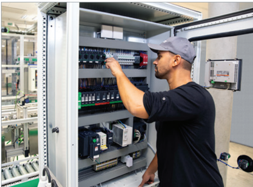
General machine control
